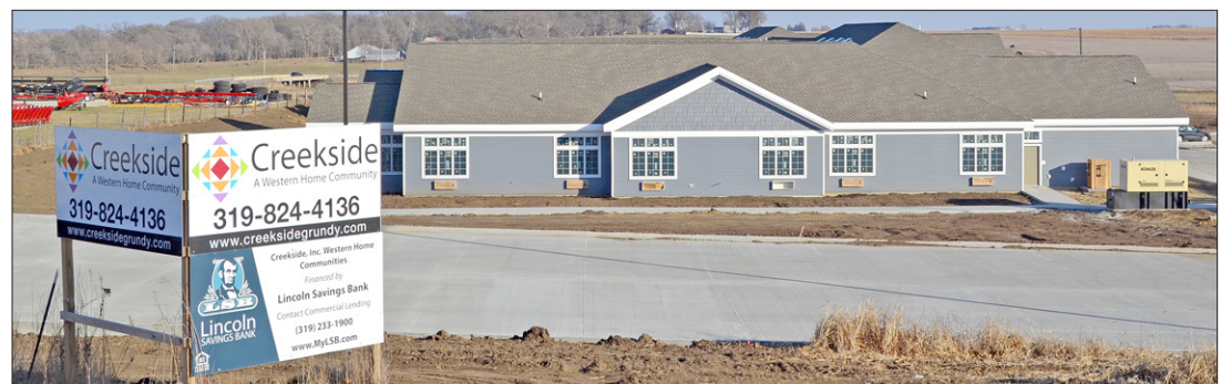
Western Home Communities' Creekside Cottages development is nearly complete on the outside, and the hope is that the new facility is finished by spring. (Michaela Kendall/The Grundy Register photo)
